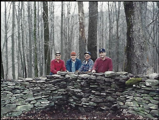
Pictured above are Robert Stanton (center) and Dave Palmer (extreme right) in approximately 1987 restoring the cemetery perimeter wall. If you know the identity of the other two individuals, let us know
